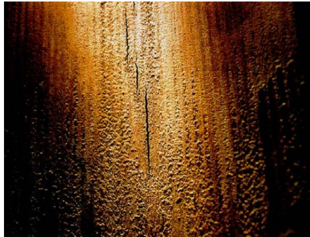
Figure 15: Chamber liner with typical longitudinal failure
